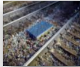
Drainage Catch Pit
